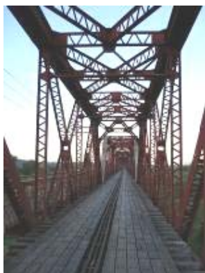
Figure 1: The railway for which this 3.6km long bridge over the Zambezi was built was destroyed during the civil war and is only now being repaired. (Photo credit: Polastro).
